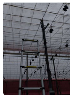
Temperature and humidity sensor positioned at the height of the cup.
