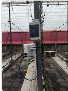
12V power supply unit installed adjacent to the datalogger.
